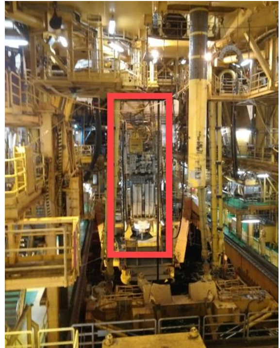
Fig. 1. WAMS setup installation area
